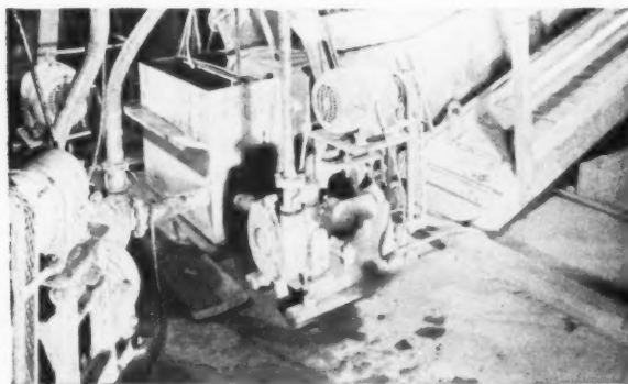
Grind Circuit Circulation Model K Pumps. These sand pumps receive the classifier overflow and pump the material to the sand slime separation circuit located at a higher elevation.
